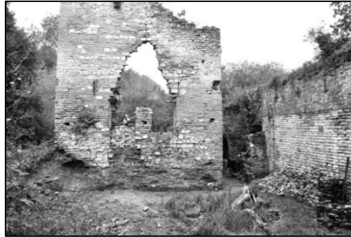
North-east wall of the Cornish Engine House at Brandy Bottom in 2011 before rebuilding by contractors.
