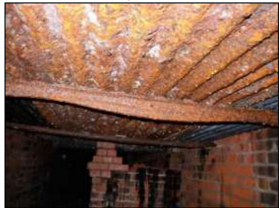
Photo 26 – View south-westwards under the floor of the Horizontal Engine House along the space between the two brick pedestals. The rusty corrugated iron at the top of the photo is the shuttering used when the modern concrete floor was cast. (© H Orr-Ewing, 2017)
