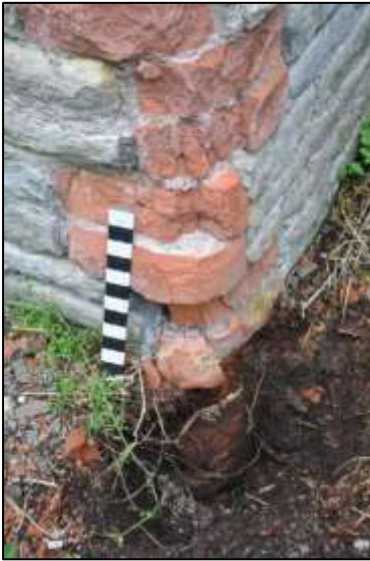
Photo 29 – Close-up of the base of the eastern corner of the Horizontal Engine House in November 2011.
