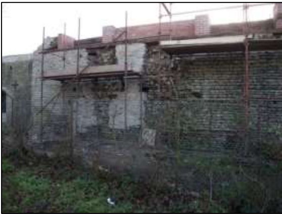
Photo 16 – View of the rebuilt north-west wall of the New Pit heapstead in mid-January before the scaffolding was taken down. The light coloured areas show where the face of the wall has been patched.
