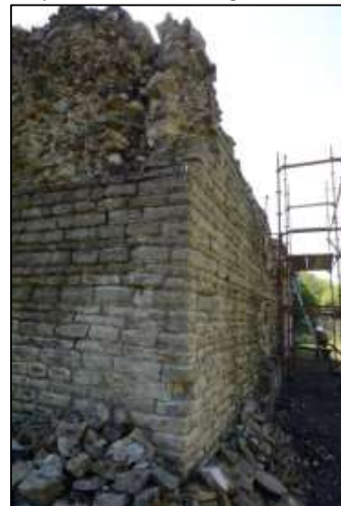
Photo 8 – Another view of the northern corner of the New Pit heapstead. The unsupported section of wall, referred to on page 1, can be seen at the top centre.
