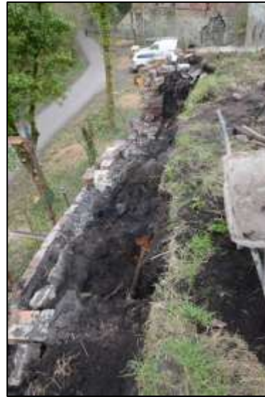
Photo 12 – The tippler slots on the north-west of the New Pit heapstead in March 2017. They had been cleared of spoil so that a specification could be drawn up for their rebuilding.
