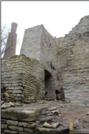
Photo 22 – ... and the wall in January 2018 after the face was patched, seen from a position below the walkway outside the south-west wall.
