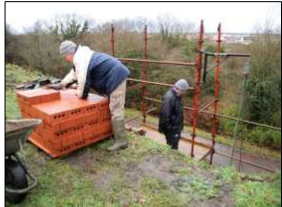
Photo 33 – Stacking new bricks on top of the New Pit heapstead ready for use in rebuilding the tippler slots.
