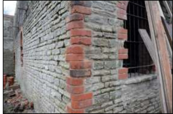
Photo 31 – The restored eastern corner of the Horizontal Engine House in January 2018. The bull-nosed bricks used came from the piles in the undercroft of the engine house.
