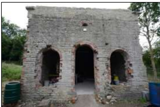
Photo 1 – The front of the Horizontal Engine House in June 2017, showing the dilapidated state of the brickwork around the door and window openings.
