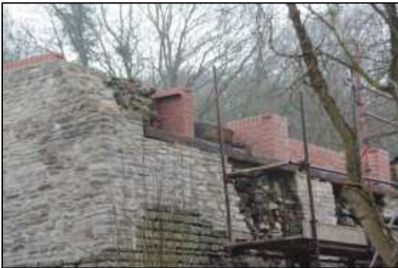
Photo 17 – Close-up of the rebuilt northern corner of the New Pit heapstead, seen from the cycle path in January 2018, during the reconstruction of the tippler slots.
