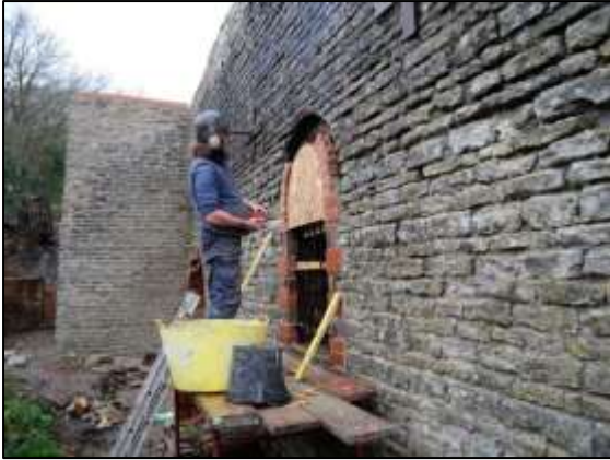
Photo 3 – A mason rebuilding the brick surround to the window in the south-east wall of the Horizontal Engine House.
