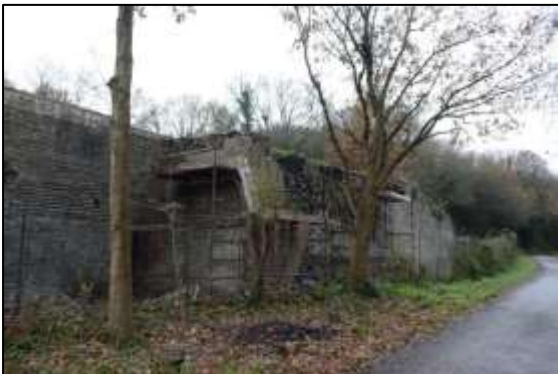
Photo 10 – The northern corner of the New Pit heapstead during the rebuilding of the vertical faces of the walls.
