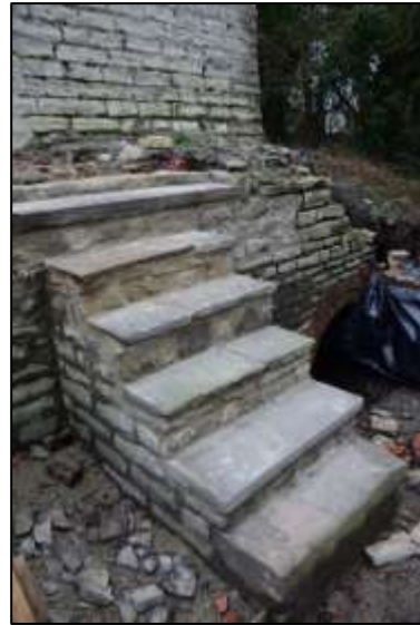
Photo 25 – ... and in January 2018 after the stone treads were rebuilt with slabs of pennant.
