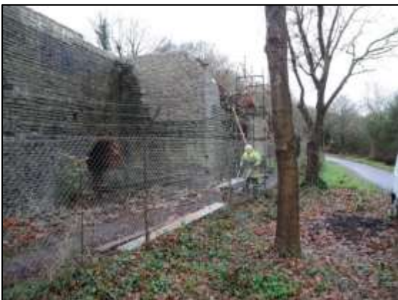
Photo 11 – The same corner of the New Pit heapstead in December 2017 after the rebuild. The light coloured areas show where the faces of the walls have been patched.
