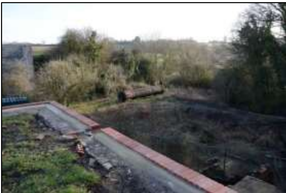
Photo 4 – The finishing soldier course of bricks has been laid along the top of the eastern corner and part of the south-east wall of the New Pit heapstead in January 2018.
