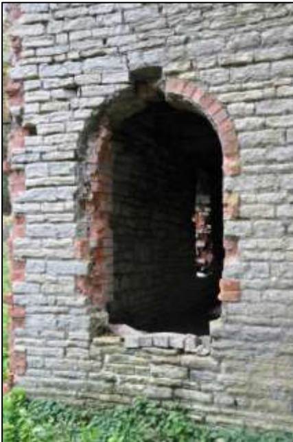
Photo 30 – The weathered state of the brickwork forming the eastern corner of the Horizontal Engine
