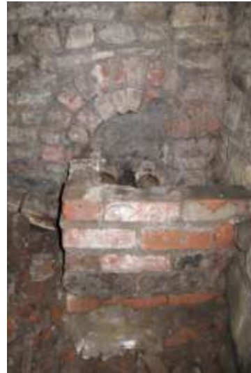
Figure 6 – Colliers' font in the undercroft of the Horizontal Engine House. © Steve Grudgings, 2013
