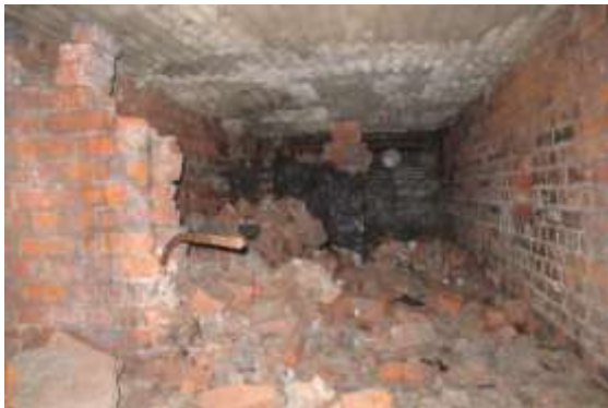
Figure 5 – View of the undercroft of the Horizontal Engine House, with grease sticking to the far wall. © Steve Grudgings, 2013
